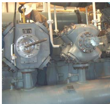
First cylinder installed next to the original cylinder. Note the discharge bottle is still in place.
