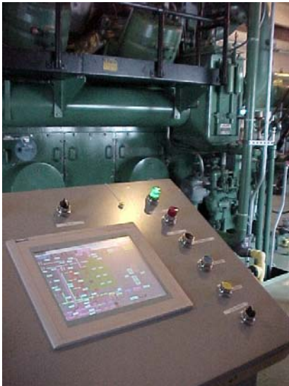
Figure-8: Local Control Panel
